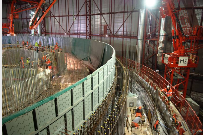
Approx. 3700 m 3 of concrete was used for both sides of the liner. This was an even larger pour than the base slab.
