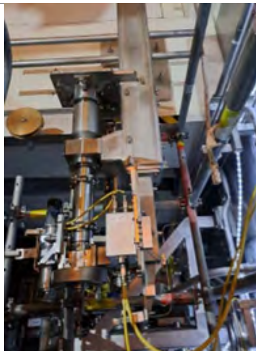
Photo 3 : potence de manutention
