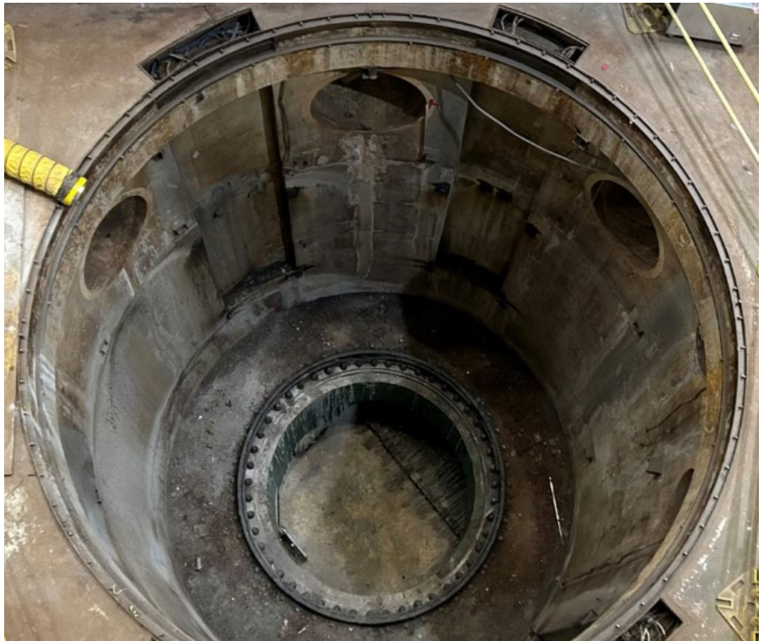
Looking down into the emptied reactor vessel cavity at Crystal River 3.
