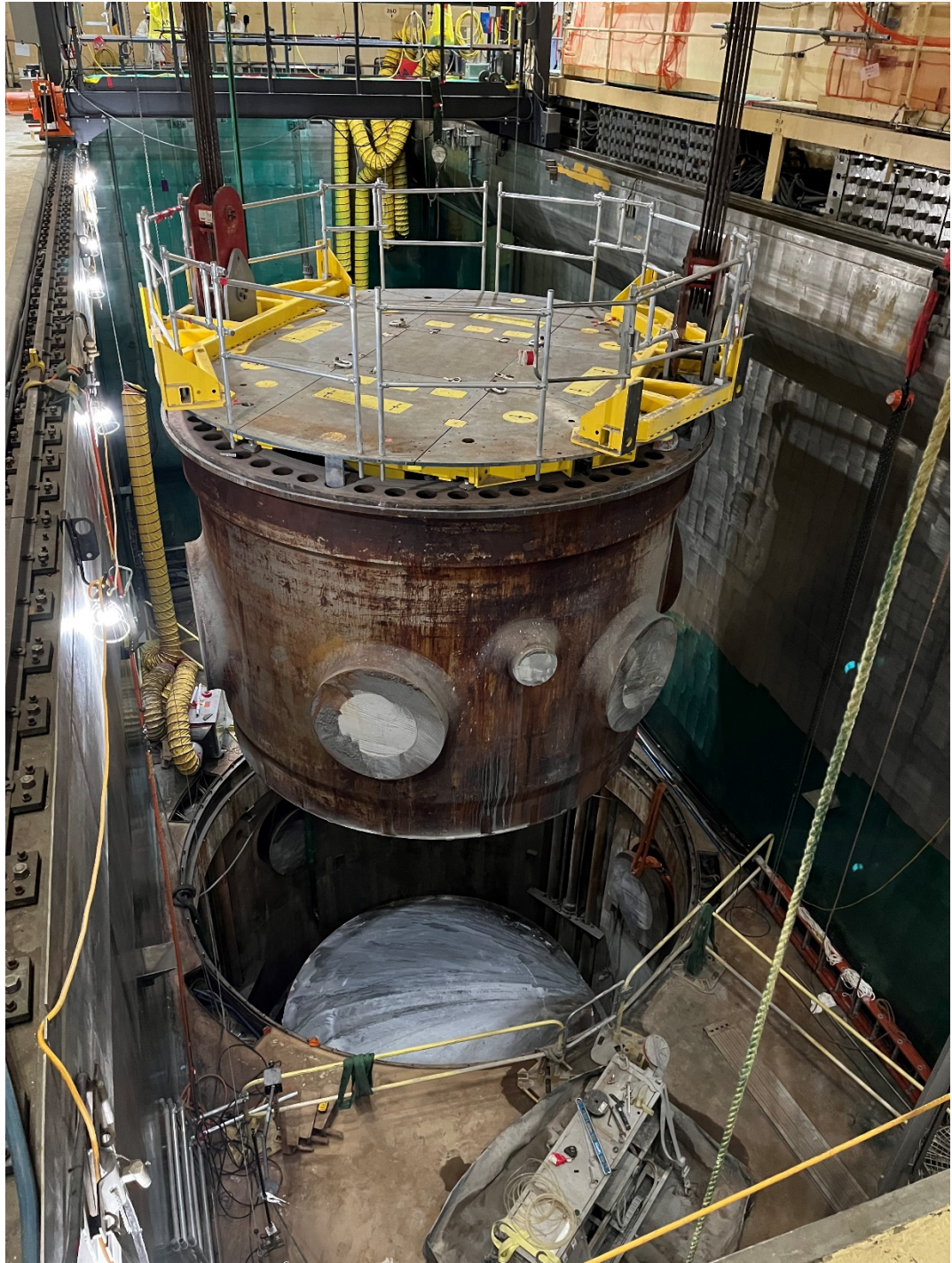
Image: Orano's team lifted the first piece of Crystal River 3's reactor pressure vessel after horizontally cutting the component and its repackaged segmented internals immobilized in solid grey grout.
