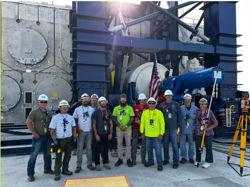
Orano Loading Crew performing the first loading of an Upper Compartment of Matrix Horizontal Storage Module (HSM).
