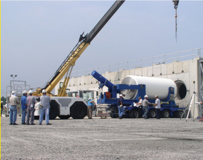
DSC (Dry Shielded Canister) being transferred to HSM.
