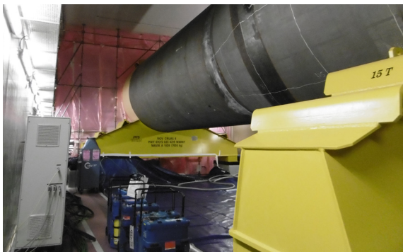
Legacy steam generator being decontaminated to meet "exempt" waste class
